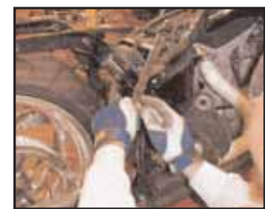
5. Mark Fender Struts and Cut off Both Sides at the Same Angle. You can re-use these later.
